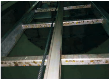
A ladder covered with oil droplets
